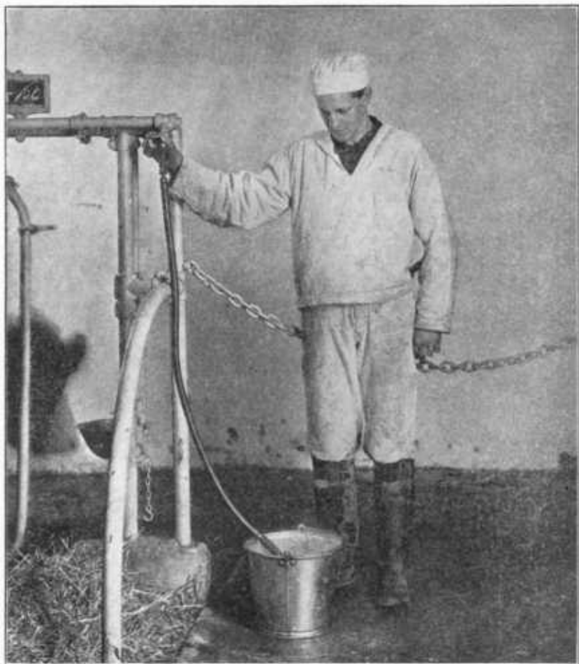
FIGURE 6.—The vacuum line should be cleaned about twice a year by drawing hot water, containing washing powder, through it with vacuum. If milk is drawn into the vacuum line, the pipe should be cleaned immediately after milking.
